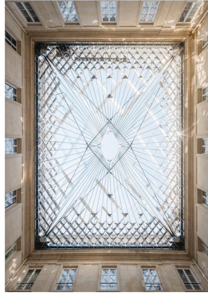
Hôtel de la marine, Glass roof of the Intendant's courtyard, Paris Designer: HDA Photo: Nicolas Trouillaud
